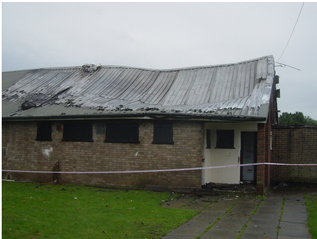
Vandalised Harold Park Pavilion 2006
